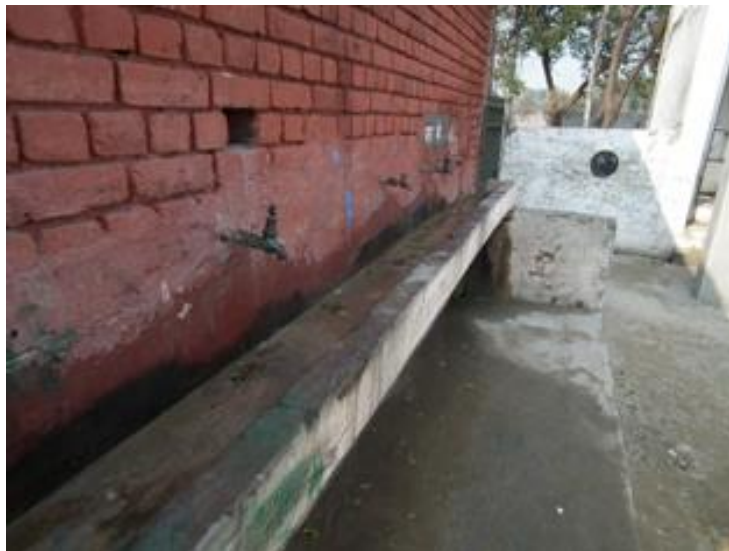
POORLY CLEANED DRINKING WATER AREA IN GSSS MAZARA DHINGRIAN
