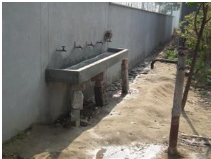
POORLY CLEANED DRINKING WATER AREA IN GSSS Nangal Khurd
